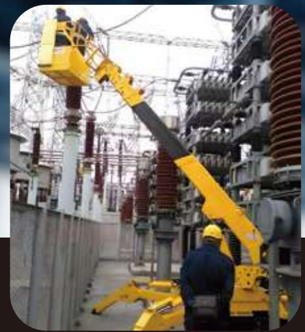
Electric power maintenance
